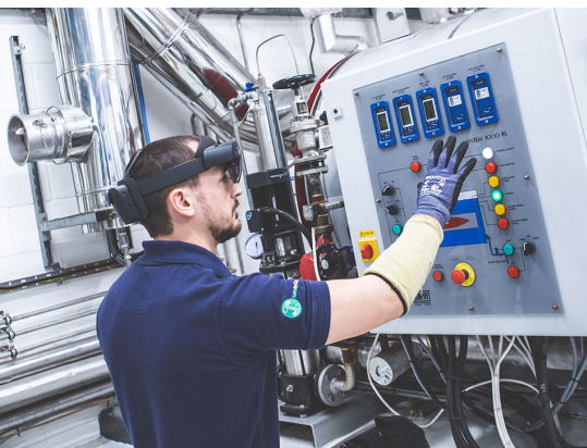
Additional Engineer carrying out steam system audit
