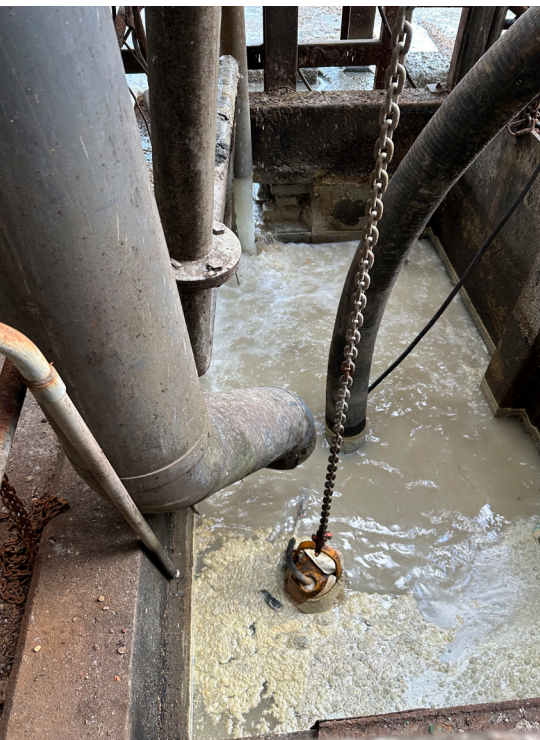
Submersible pump in-situ
