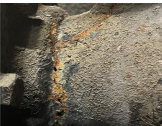
Split in the outlet pipe
