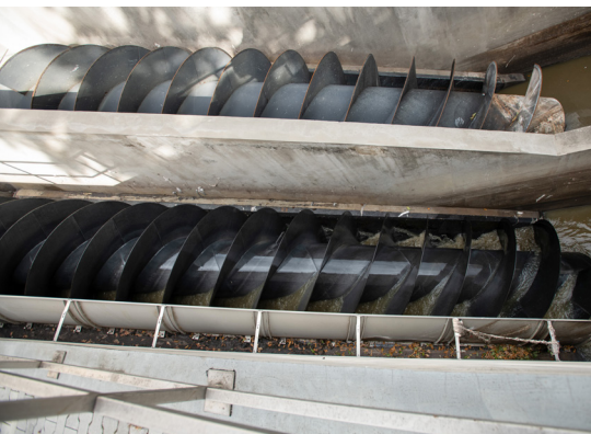
Two archimedes screws tasked to remove water from the effluent pit
