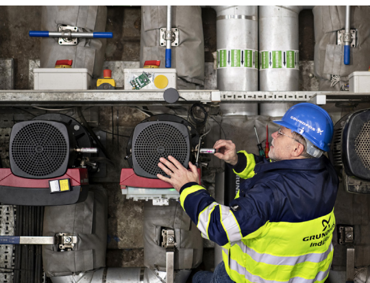
Grundfos Senior Application Manager at one of the new CRIE pumps for the boiler feed level control
