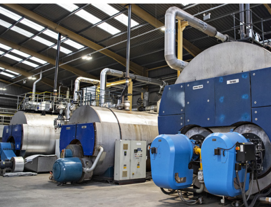
Three of the steam boilers at the Distillery in Scotland
