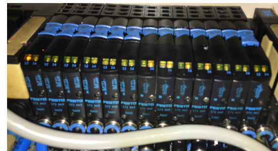
Newly installed, updated solution
