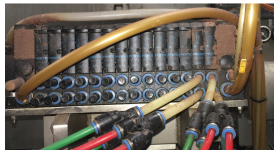
Obsolete manifold solution
